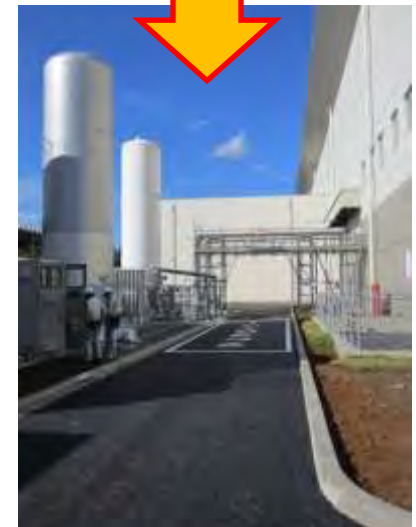
Tilted liquid He tanks were straightened. The surrounding road was also restored.
