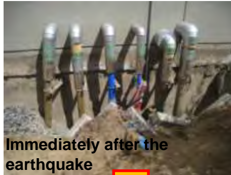
Piping system around the building was heavily damaged.
